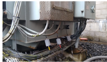
Fig. 10: Acoustic sensors mounted on a tank wall
