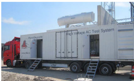
Fig. 1: Mobile transformer test system, 1.3MW
