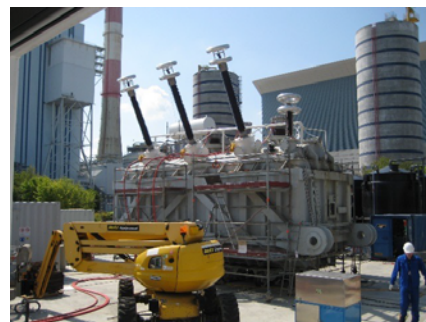
Fig. 6: Preparation for an induced voltage test
