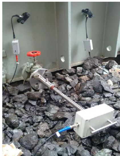
Fig. 8: Transformer valve sensor (TVS2)
