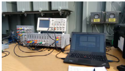
Fig. 12: On-site test setup with the ICMsys8
