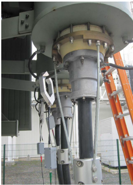
Fig. 9: Clamp-on HFCT fitted to a cable bushing
