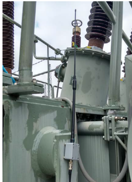
Fig. 14: Disturbance antenna DA1
