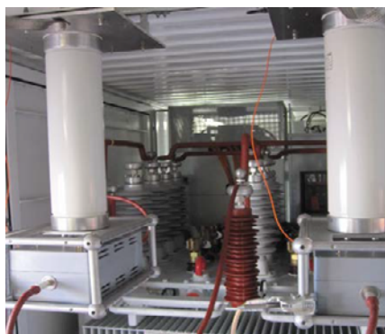
Fig. 4: HV filters with embedded current transformer and capacitive voltage divider
